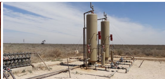
Water and chemical flow monitoring at oil wells
